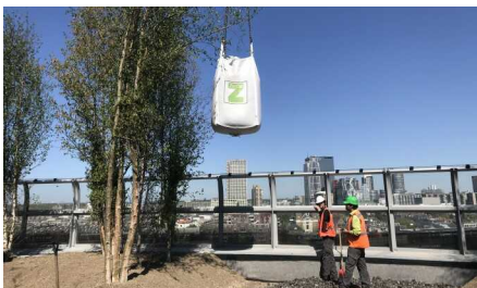
The substrate and the trees both are lifted on the roof with a telescopic crane.
