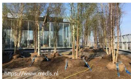
The root balls are anchored to the ground to withstand the high wind loads on the roof.
